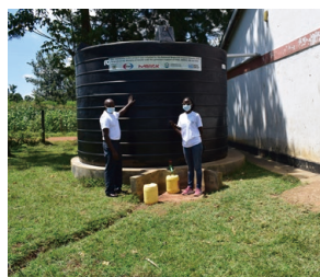
The tanks installed next to local schools
